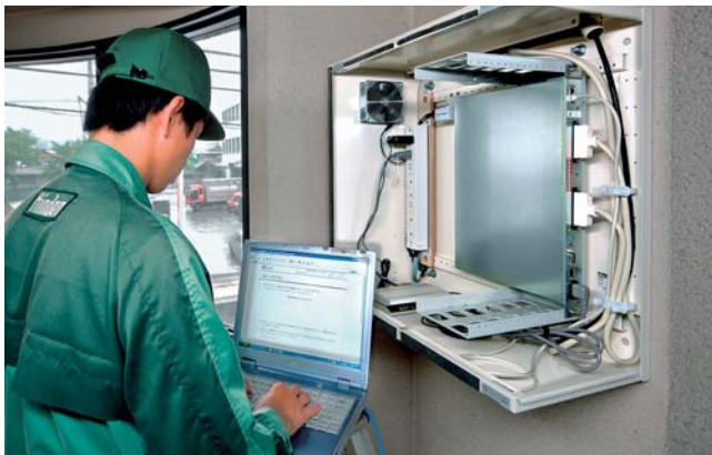
Information & Communications Network Installation work on eo Hikari Net Condominium type of K-Opticom Corporation (Nara)
