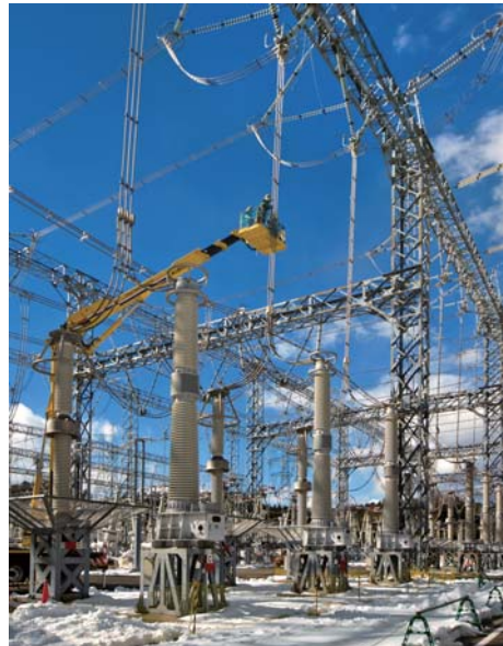
Electric Power & Others Power substation of The Kansai Electric Power Co., Inc. (Kyoto)
