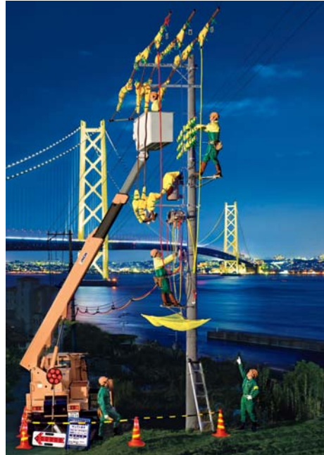
Power Distribution Lining Installation work on power distribution lines of The Kansai Electric Power Co., Inc. (Hyogo)
