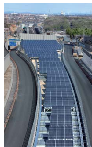
Solar power generation facilities at Nagoya-Daini-Kanjo Expressway
