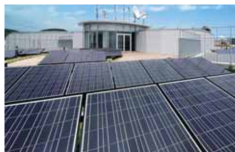
Solar power generation facility at the Iwakuni City Hall, Yamaguchi Prefecture
