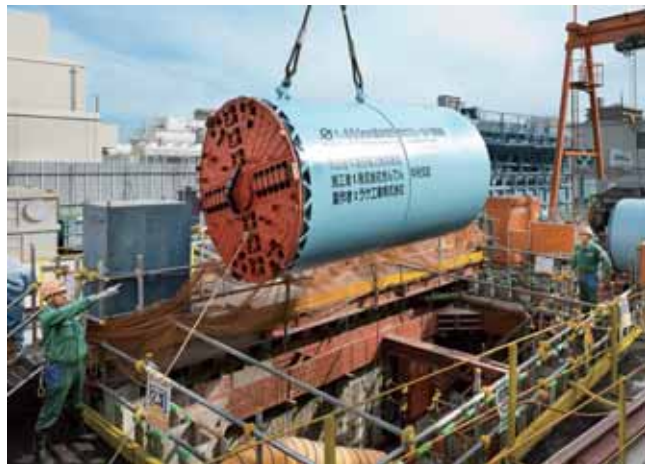
Electric Power & Others Underground power transmission lines at Sakai port (Osaka): Underground power transmission lines
