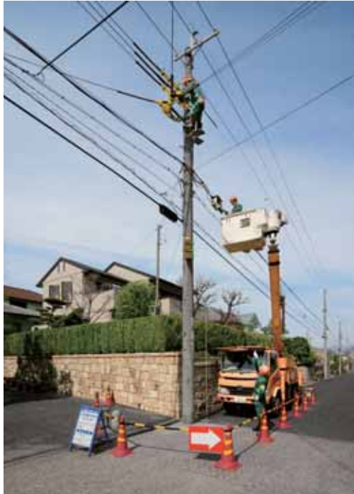
Power Distribution Lining Installation work on high-voltage power distribution lines to ensure uninterrupted power supply (Hyogo): The Kansai Electric Power Co., Inc.
