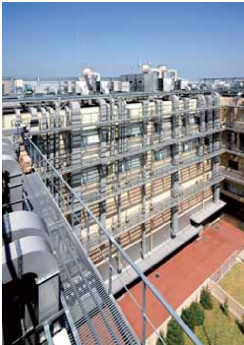
Environmental Management Facilities The School of Life and Environment Science, Osaka Prefecture University (Osaka): Air-conditioning systems and sanitary plumbings
